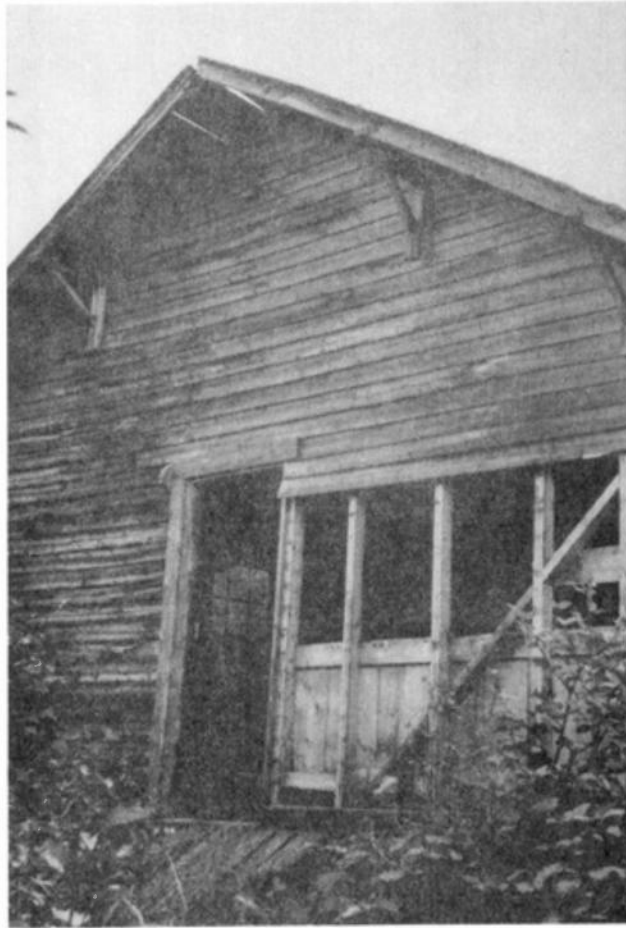
Plate 58 — West building, north end, in 1977 just before it was destroyed. Note where siding had been taken off. (BLM photo.)
