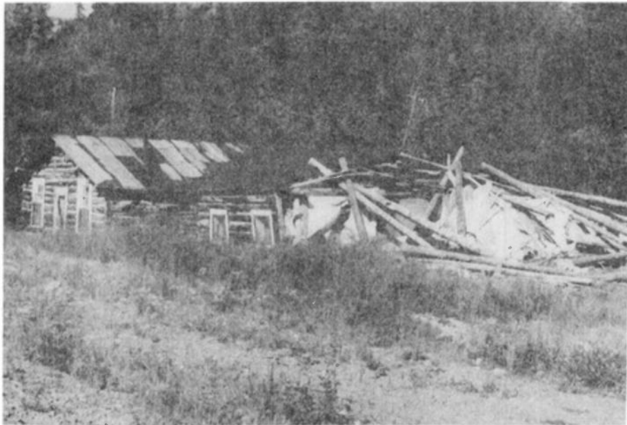
Plate 75 — Paxson Lodge in 1977. Fire destroyed more than half of the H-shaped building Christmas 1975. (BLM photo.)
